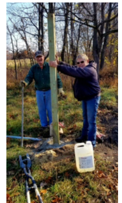
Prairie Trails Club volunteers installed an equestrian hitching rack so users have a way to rest their horses on a grassy spot near the trail at 700E.
